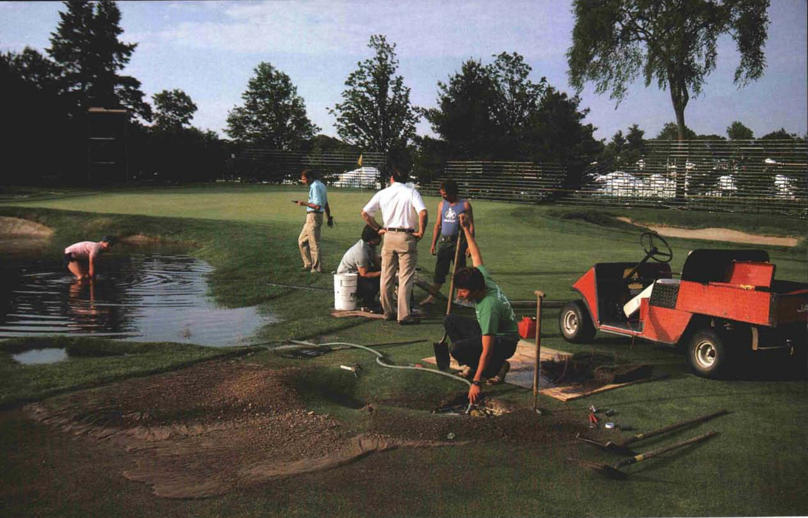
A water line break demands quick attention just before the championship begins.
