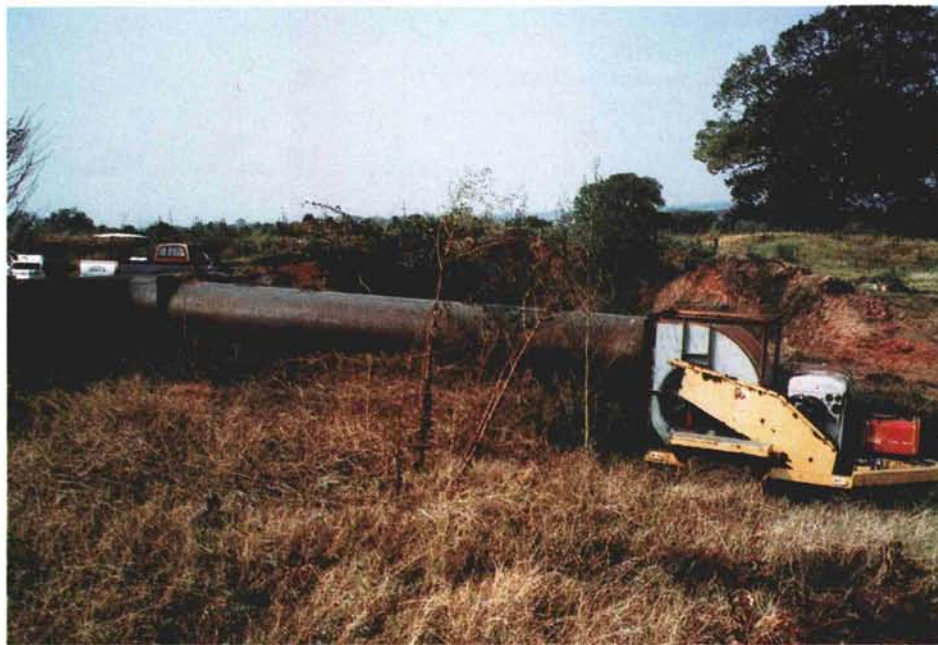
Constructing a forced-air incinerator for burning brush solved Southern Hills Country Club's problem of what to do with an overabundance of tree brush after an extensive tree improvement program was implemented.
