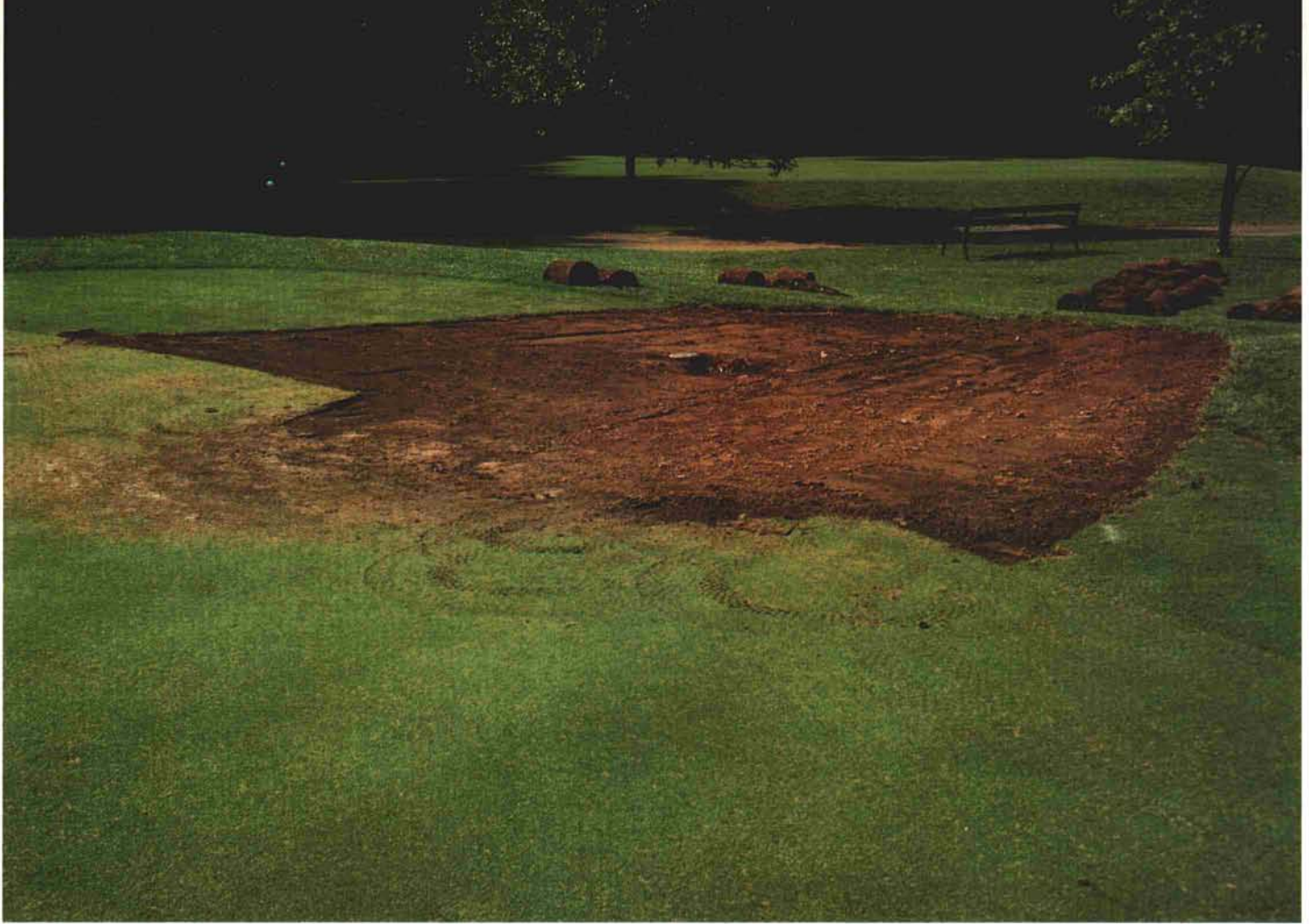
In this instance, poor surface drainage was corrected by removing the sod, regrading the soil, and replacing the sod.
