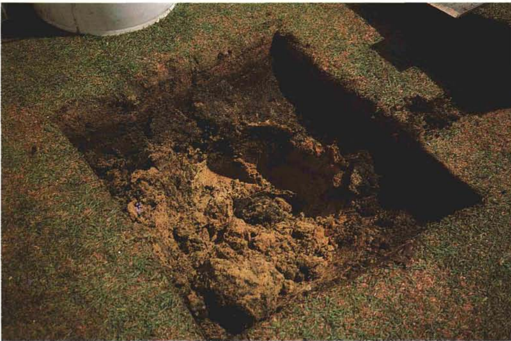
On-site mixing failed (Colorado, 1986)
