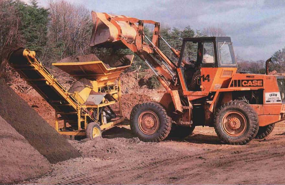
(Left) An off-site mixing operation using a front end loader and Lindig soil mixer.
