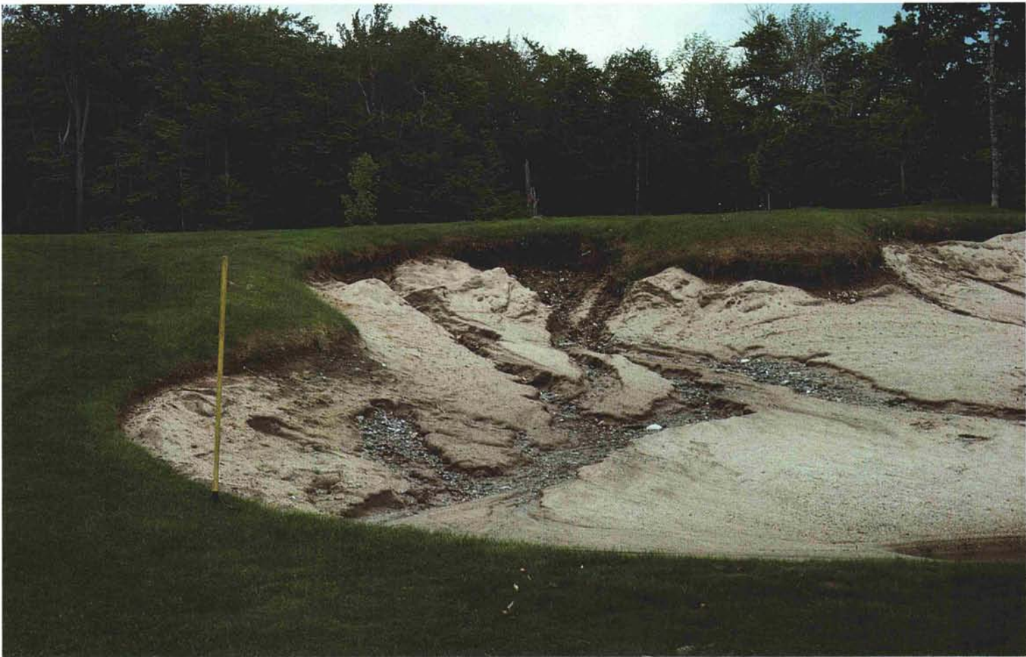
Severe washouts (above) can be reduced or eliminated with the construction of interceptor drains (facing page) or surface swales.
