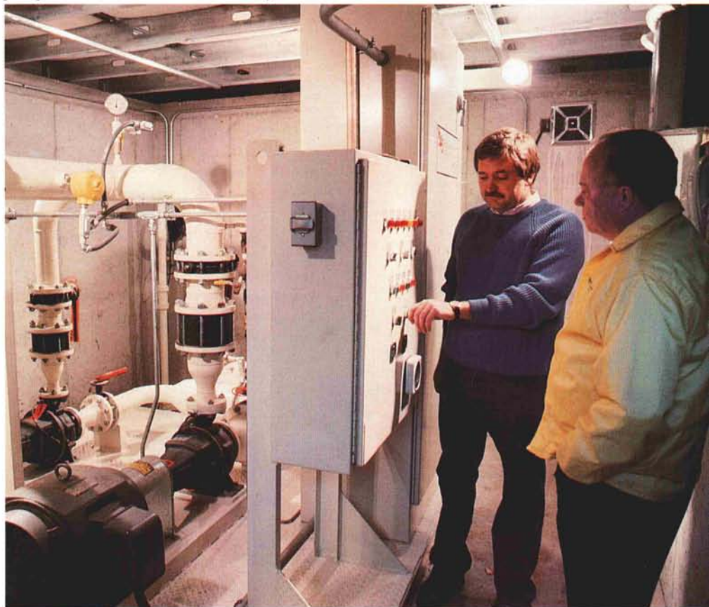
Ed Huggins and Jack Robinson looking at their new pump station. The newly installed VFD pump station at Indian Hills Country Club.
