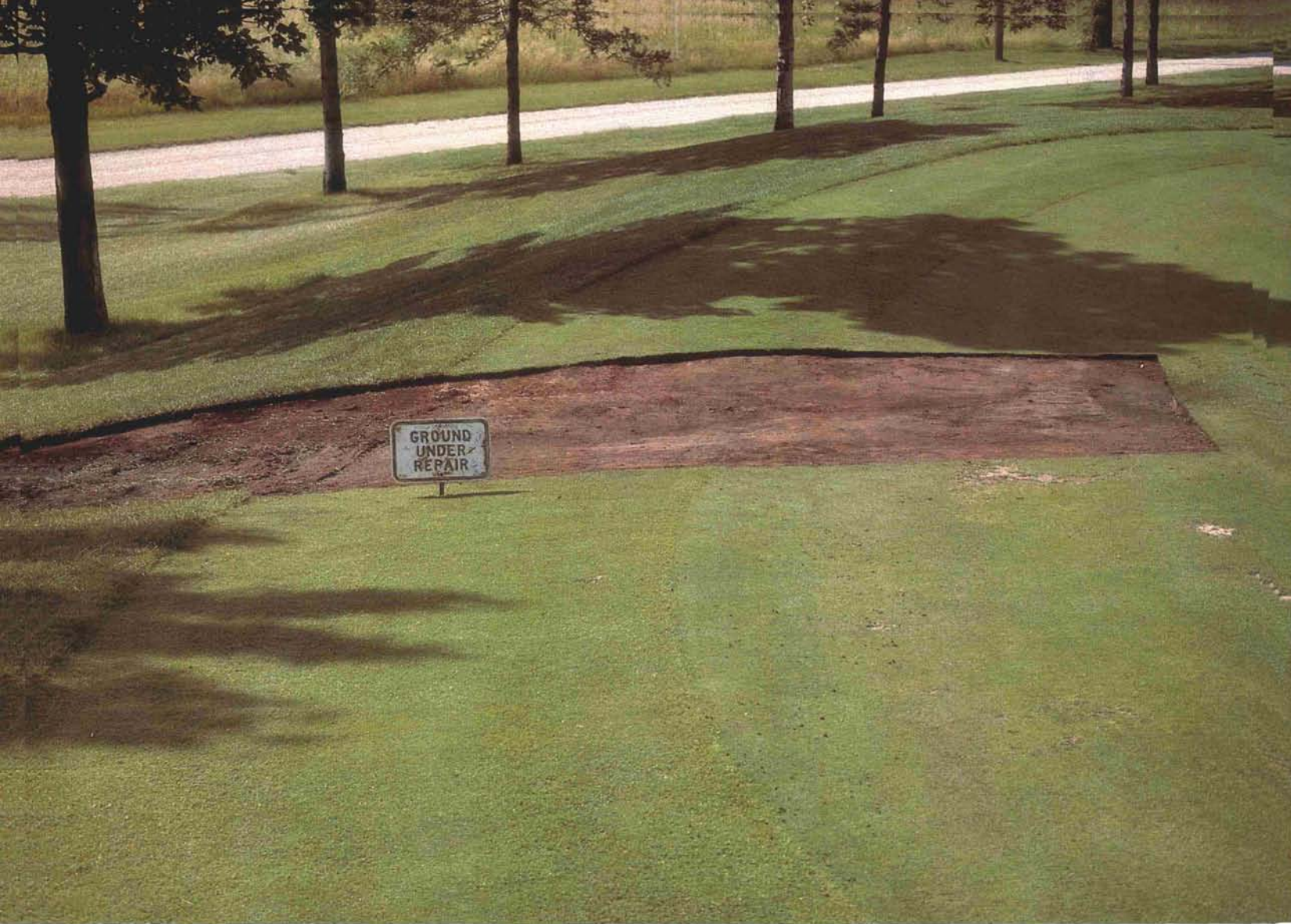
Figure 5. Recontouring an area to provide better surface drainage, eliminating a low spot which holds ice in winter and water on the surface in the summer. Both spell trouble.
