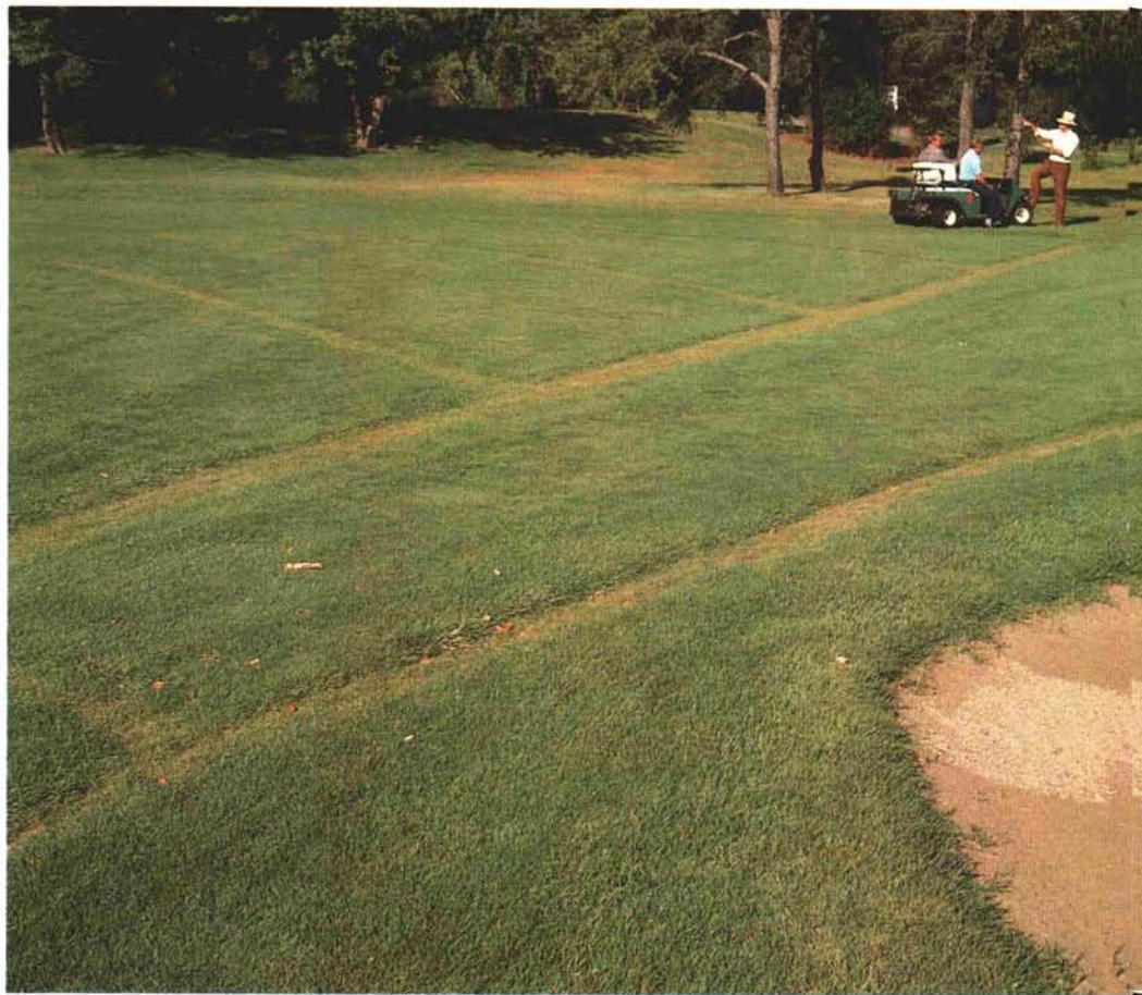
Good drainage is a prerequisite for good turf. Tile and stone-filled trenches are topped off with coarse sand and then seeded at Cherry Hills Club, Ontario, Canada.
