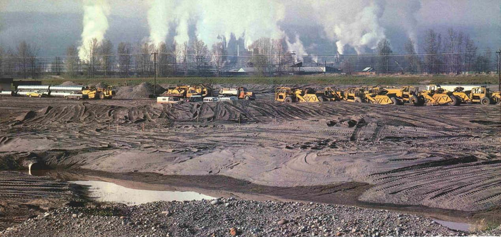
Some of the earth-moving equipment and haul-road culvert used during rough grading for the Kelso course.
