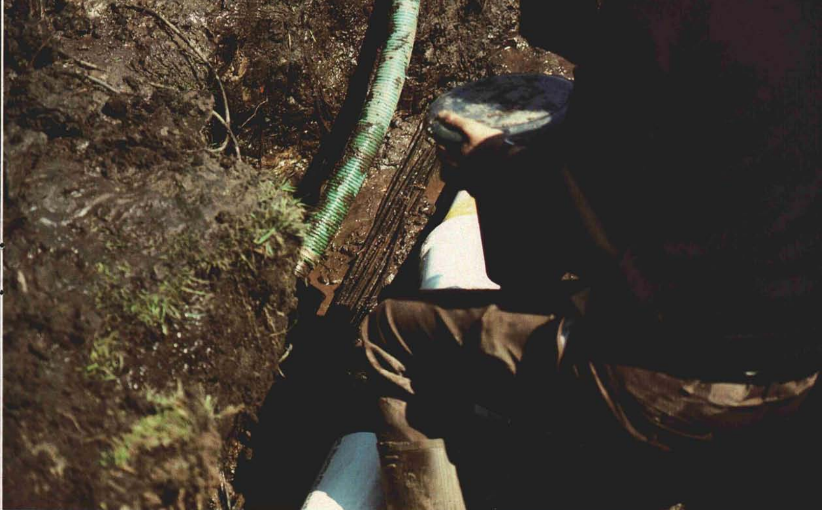
Bundled control tubing makes for easy repair.
