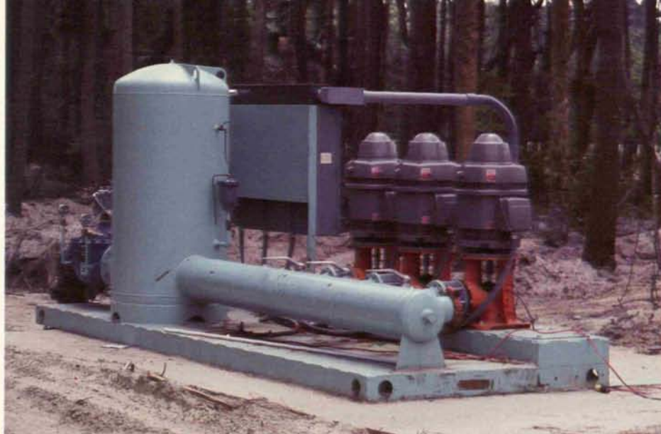
Pump selection is important. Energy requirements differ for turbine vs. centrifugal vs. submersible pumps.
