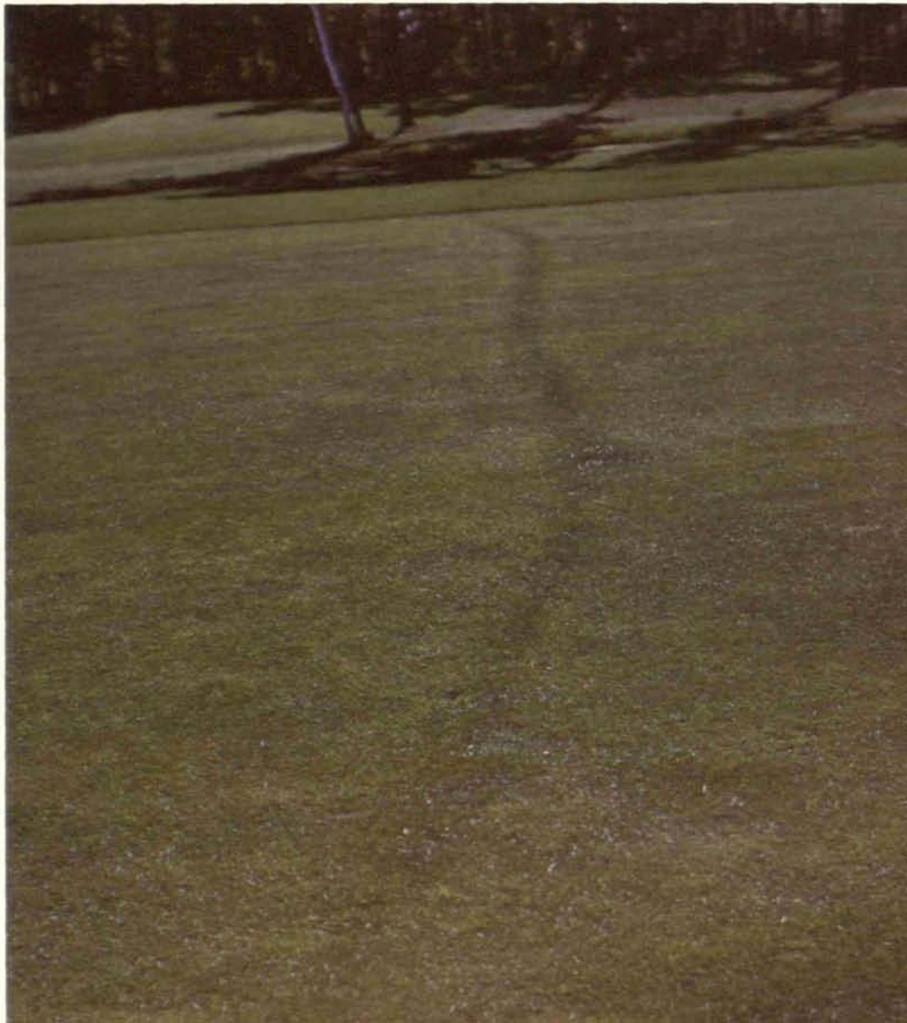
Figure 3. Turf eventually grows over the stone, but this does not impair the effectiveness of the drainage system. Twin Hills Country Club, Massachusetts.
