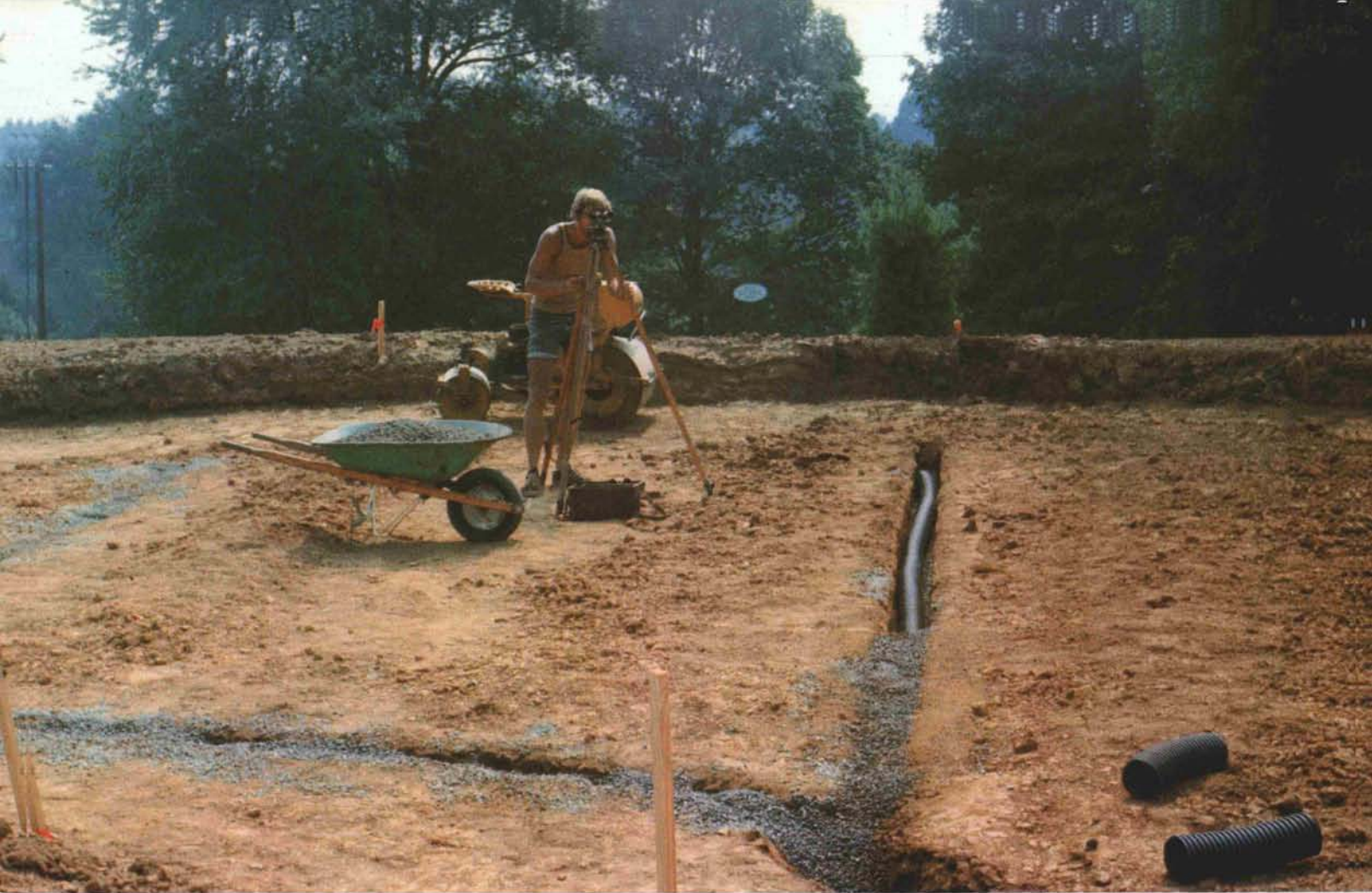
Perforated plastic 4-inch tubing serves as drain line. Worker covers drain with gravel.
