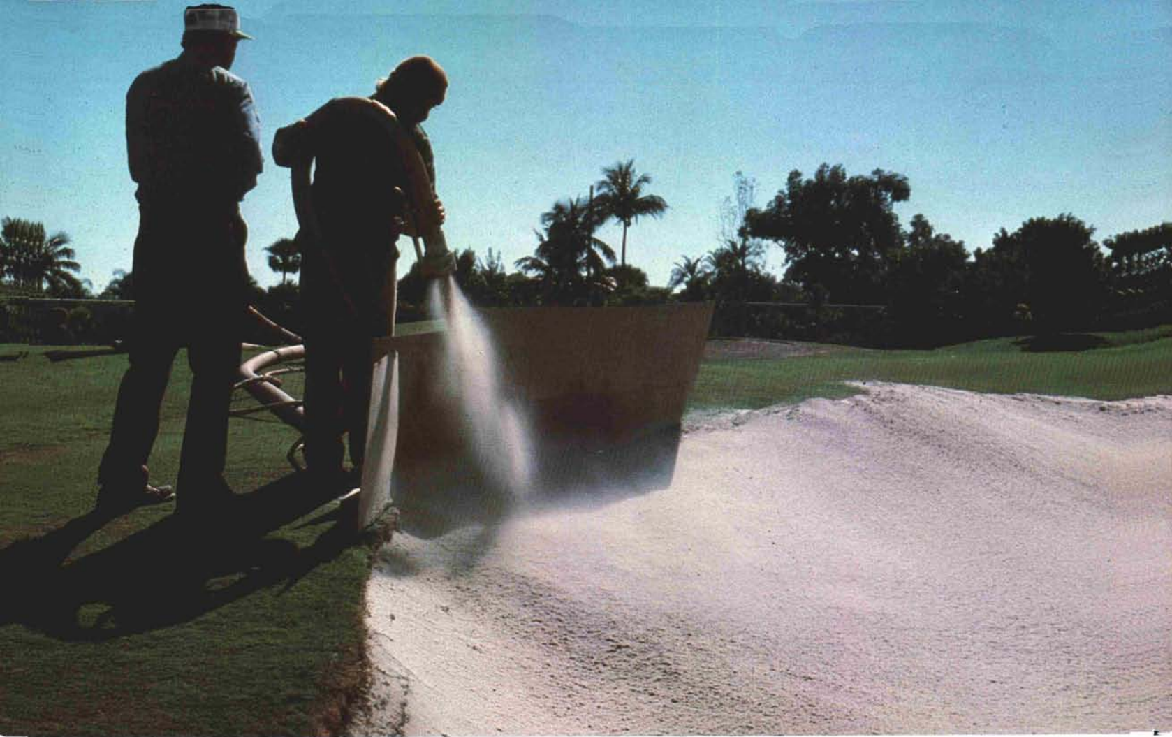
The gunite method compacts the sand in place. The plywood board keeps sand within the bunker.
