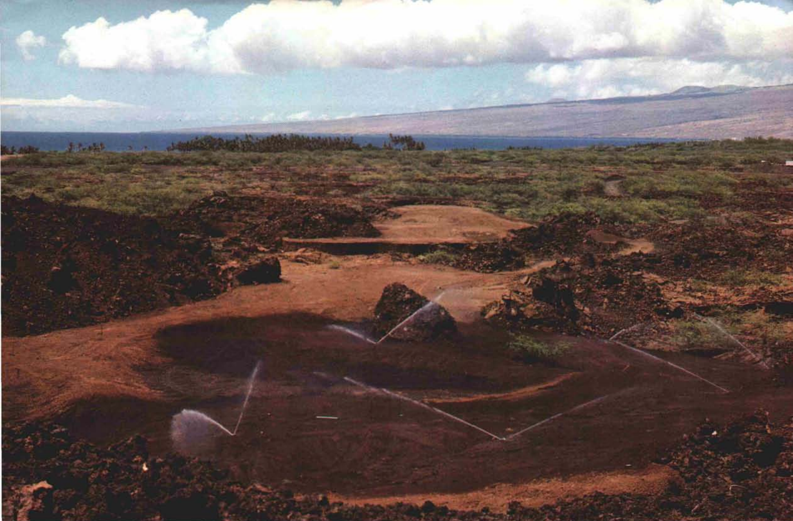
New Mauna Loa golf course, on the island of Hawaii, is being constructed on a base of 100-year-old lava.
