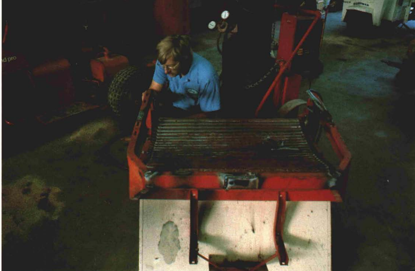
Traction bar is bent and welded across front of hopper.
