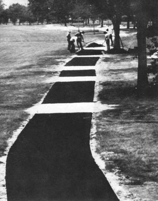
John Biddy at Lakeside Country Club, Houston, Texas, placed concrete in low drainage areas for minimum repair.
