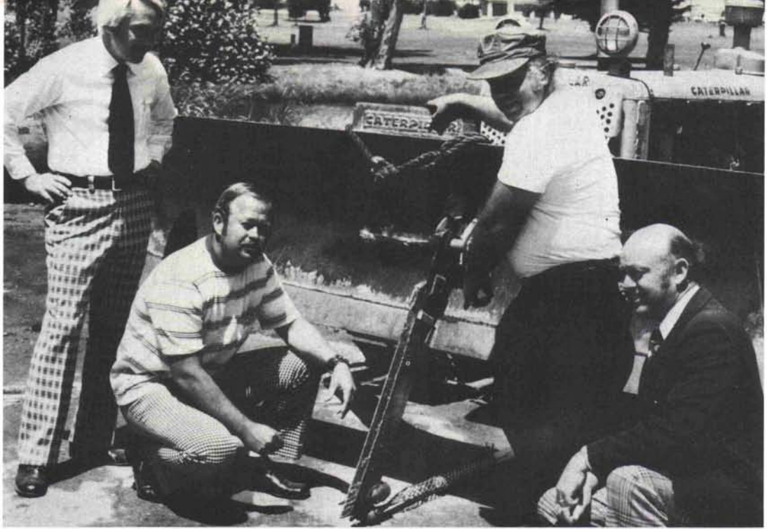
The Team (left to right, R. Harrison, D. Plato, G. Acia and G. Mainland) and the pipe puller at Alameda.
