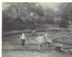
COVER PHOTO—Installing drain lines in the sub grade of a putting green.
