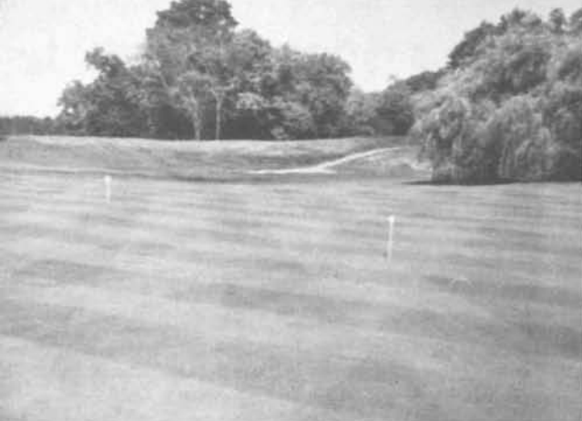
Matured soil nursery, prepared in advance of actual green construction using the same soil to desired sub-grade.
