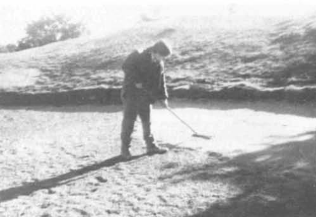
Coarse sand layer being installed over the stone base continues to be an integral part of the construction procedure.
