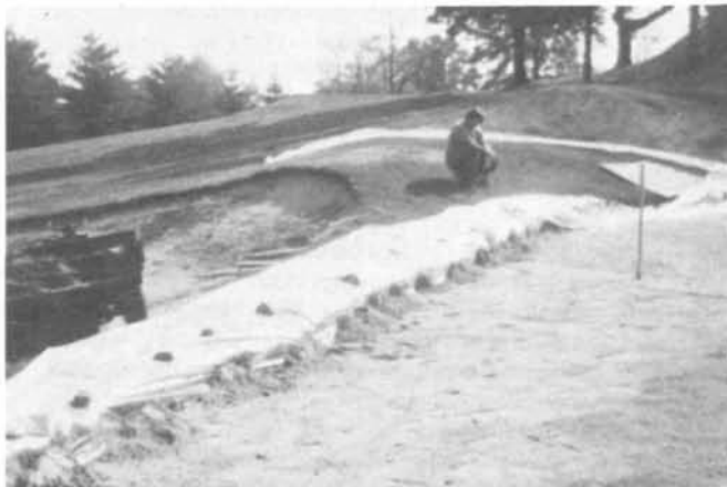
Ringing the green with plastic as an interface between native soil and new greens soil.
