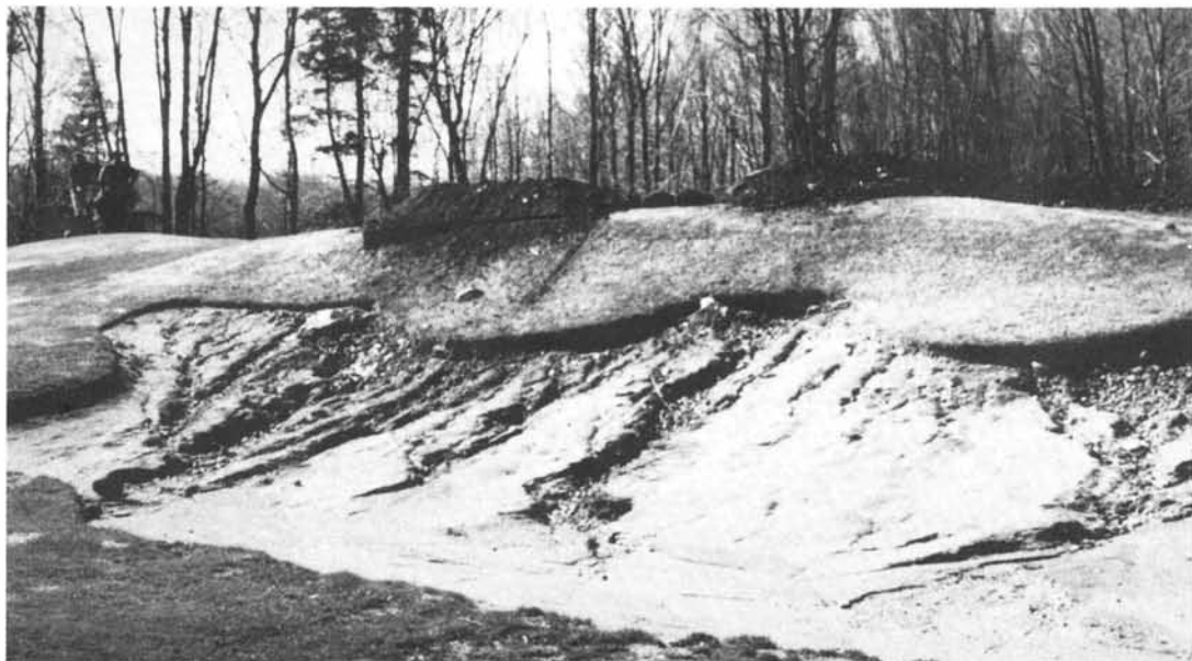
Surface runoff causes erosion and shoveling problems.
