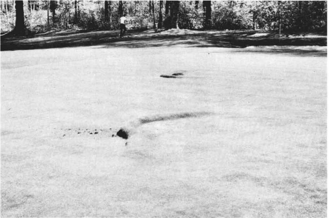
Many factors can cause shallow rooting in turf, especially poor watering practices and a soil which has inadequate drainage. In this case a water leak from an irrigation valve in the center of the green separated the turf mat on top from the roots below. The turf rolled up like a rug.
