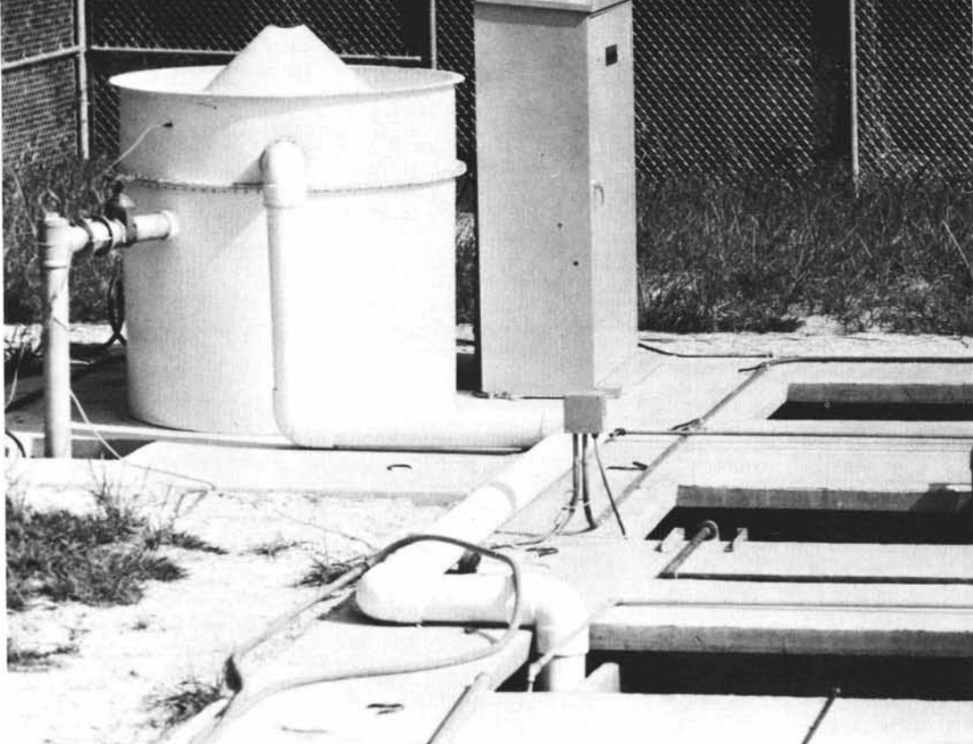
Defiance Sewage Treatment Plant with filtration system located at Atlanta Athletic Club where filtered effluent is used in the golf course irrigation water.
