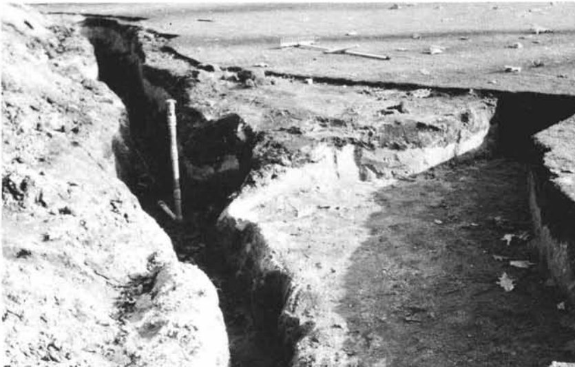
During construction the sand and topsoil were not mixed.
