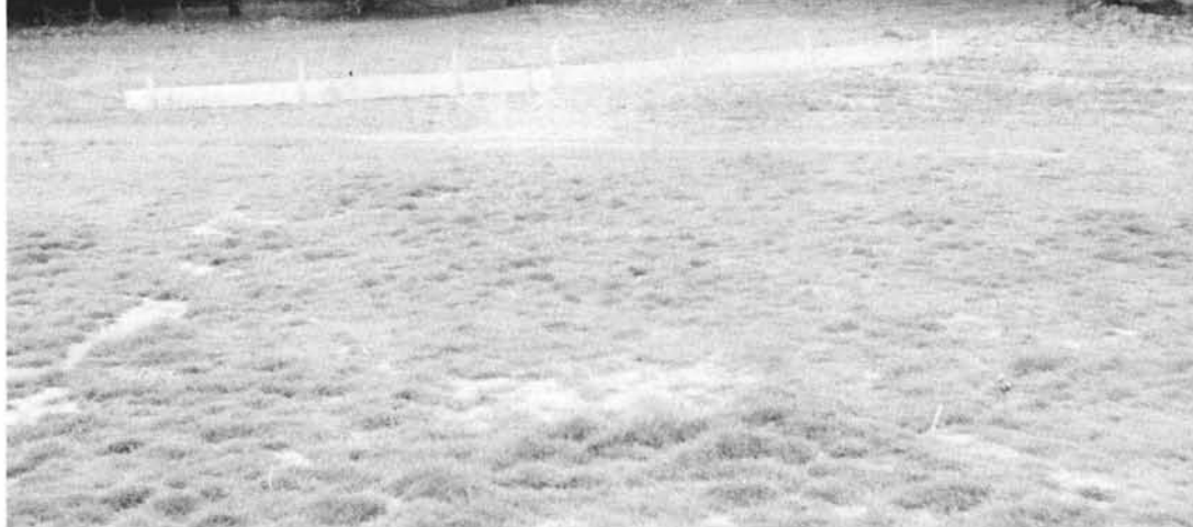
When erosion started during construction, the area was not regraded; boards were placed to divert water. What happens when boards are eventually removed?
