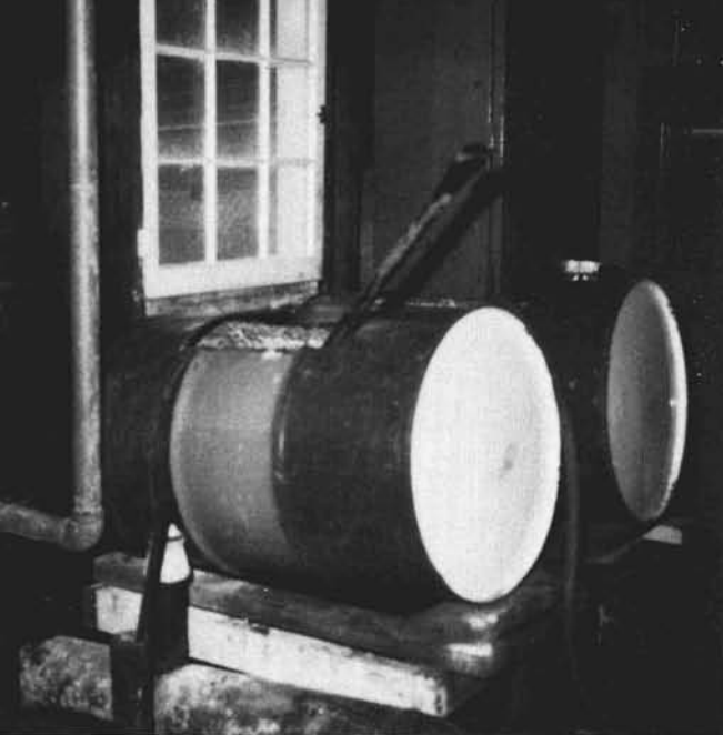
Two 50-gallon steel drums where water and fertilizer are added in the pump house.
