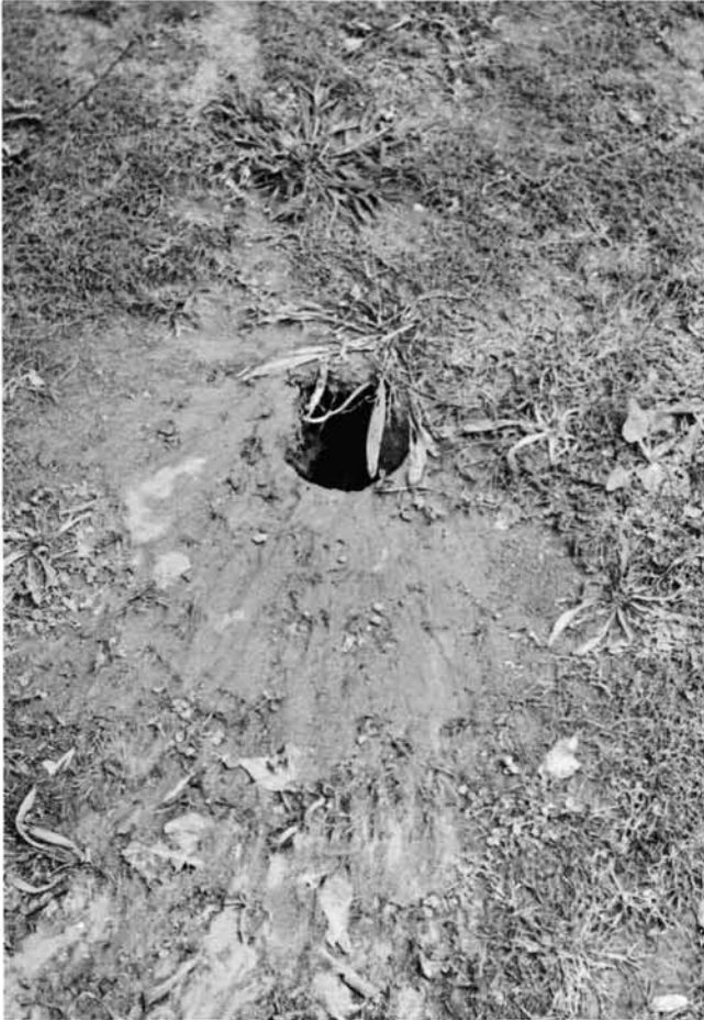
from installing a drain from the center of the bunker (left) where the first rain caused a blowout.
