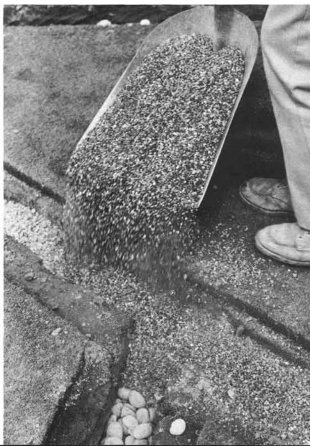
Backfilling the drain lines with graded gravel to be followed with sand. The original sod (with a sand base) will then finish the job.
