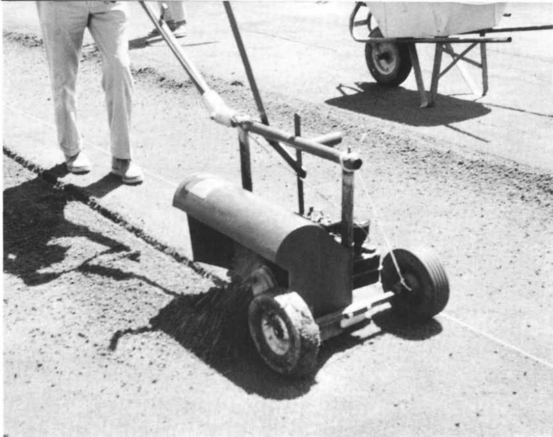
Putting green slots being cut with a modified commercial trencher. This was more effective than the chain saw method.
