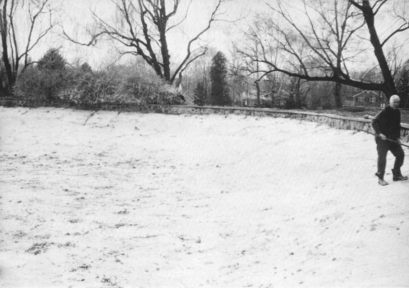
This is the base of the pond after the bentonite was completely spread.
