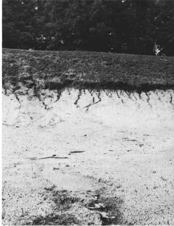
Rains cause sand erosion on slopes.
