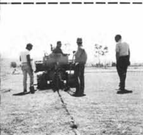
Cover Photo: A time-saving and neat job of installing automatic irrigation systems is possible by the new technique of "pulling pipe" through the ground without need for digging ditches. This "instant" way to course watering with flexible pipes is one more innovation in the trend toward complete irrigation of golf fairways. See the article by John H. Madison on automatic irrigation starting on Page 10.
