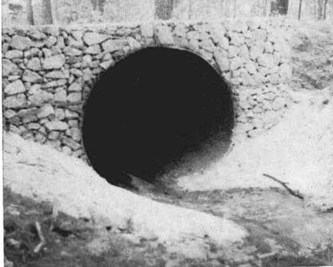
The beginning of the 640 feet of the 84" metal drain pipe laid at 2.5% grade with two reinforced concrete catch basins.
