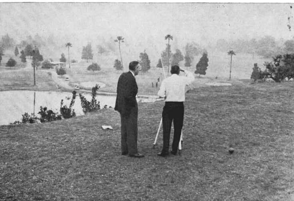
There is only one way to measure a golf hole of this kind accurately. The steep bank and lake below make the use of surveyor's instruments mandatory.
