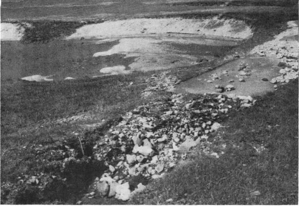
Erosion problems are accentuated at beginning of hardtop paths. Car, cart, and foot traffic wear the turf and a minor erosion problem could quickly develop into something big. Path leading away from No. 7 green at Woodbride Country Club, Woodbridge, Conn. the day after a heavy rainfall.
