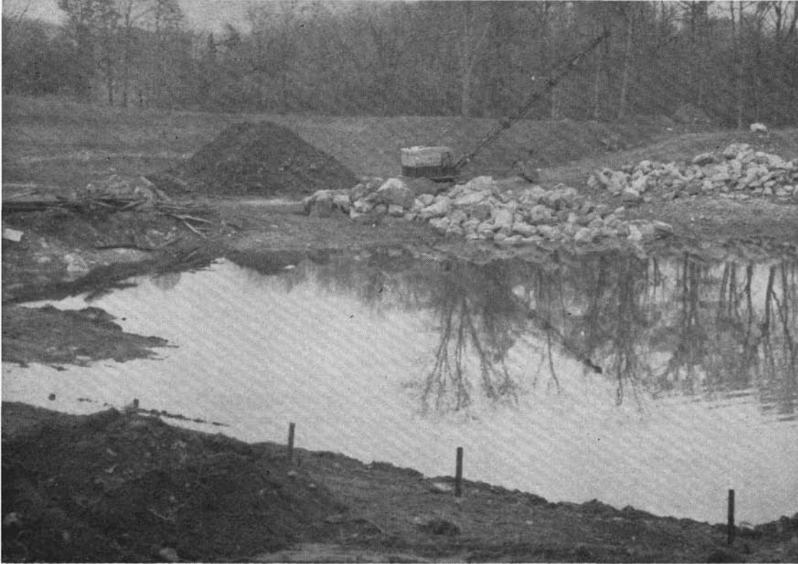
Woodway Country Club, Darien, Conn. Lake construction designed to contain 30 million gallons of water.
