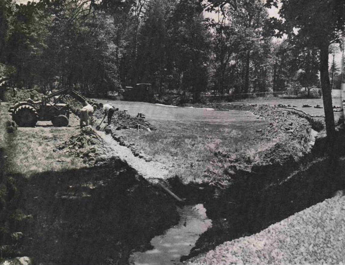
The job at Congressional is nearly complete. Tile has been installed, the gravel backfill is in place. Now a small amount of soil will be replaced and the sod laid back and tamped smooth, ready for the Open.
