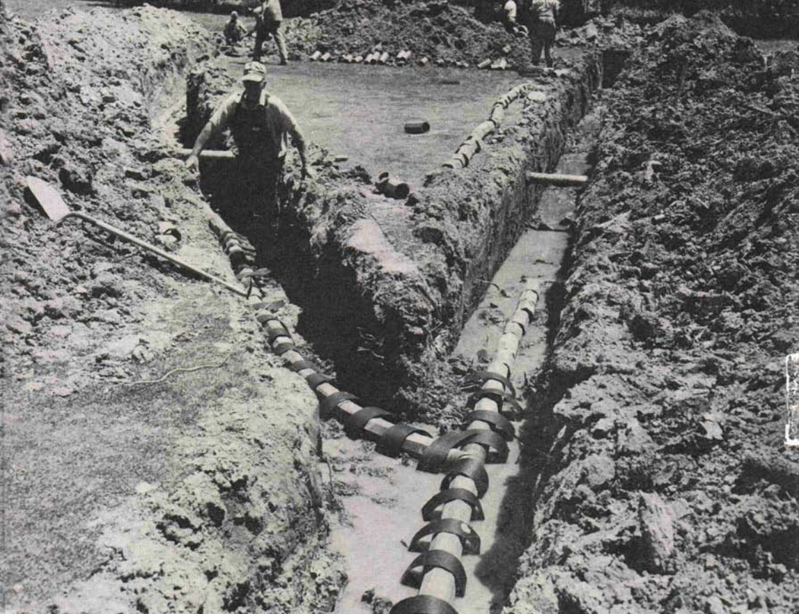
Tiles are being placed to effect rapid removal of water seeping into the trench. Note the strips of tar paper which were to be used to cover the joints, thus keeping gravel or soil from falling into the tile line. Note also the abundance of tree roots growing out from the sides of the ditch.
