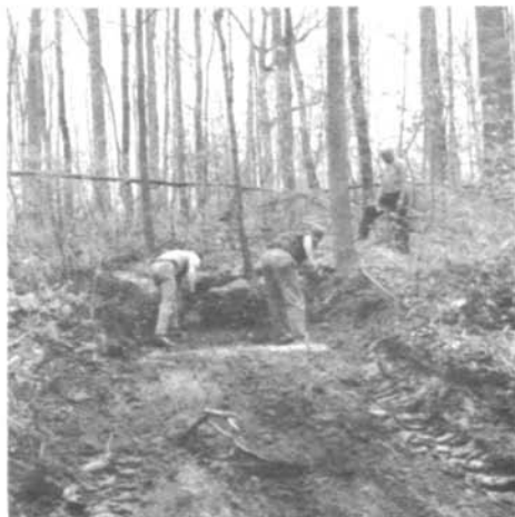
2. The rough digging is done by a front end loader or backhoe. A minimum of fine work with pick and shovel is required. The tree is selected from the wooded area on the course.
