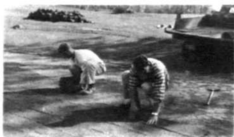
3. Matching the sod and tightening the joints. Note truck stops on apron.
