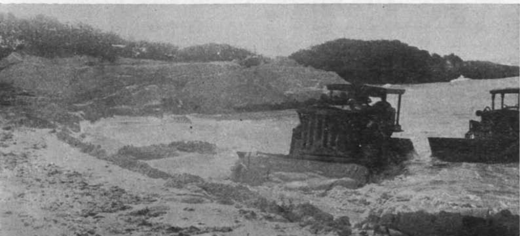
Bulldozers take to the water when it comes to grading a green in the ocean. The course in question is on Eleuthera, in the Bahamas, designed by Robert Trent Jones.
