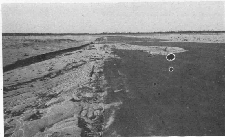
Result of lack of grass cover on airfield. Note the soil which has been washed onto the runway from adjacent bare areas. Such a condition might be prevented if a good grass cover were established.
