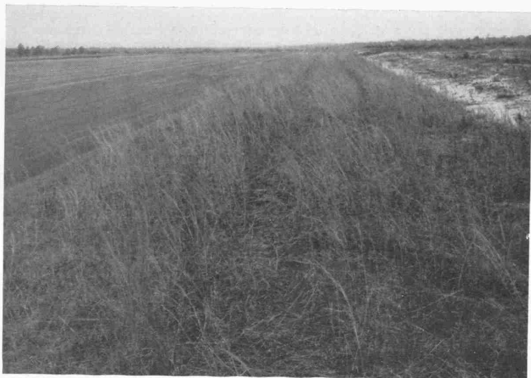
Ten-foot strip of muck which has been in place along edge of airfield runway approximately one year. Note the dense growth of natural vegetation on this strip which prevents soil from washing onto the runway. Often the vegetation obtained in this way will not survive the dry conditions on airfields since it is usually brought in from low swampy areas.
