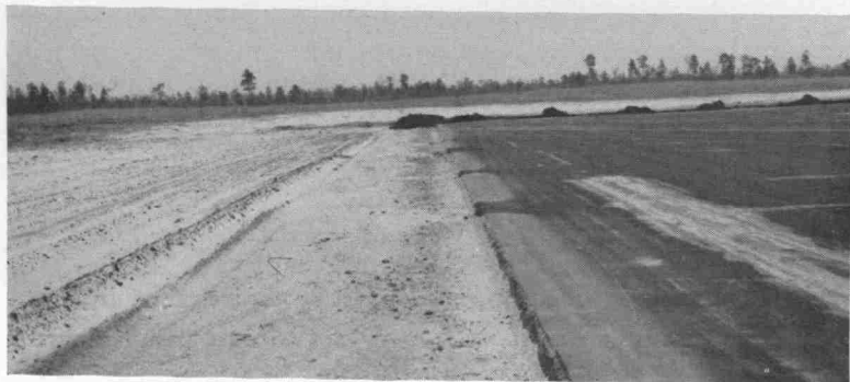
Trench 10 feet wide at the edge of an airfield runway excavated in preparation for "mucking." A 4 to 6-inch layer of muck is used to fill the trench. Natural vegetation growing in the muck is expected to produce a dense cover along the edge of the runway. The muck has already been placed in the trench in the background.
