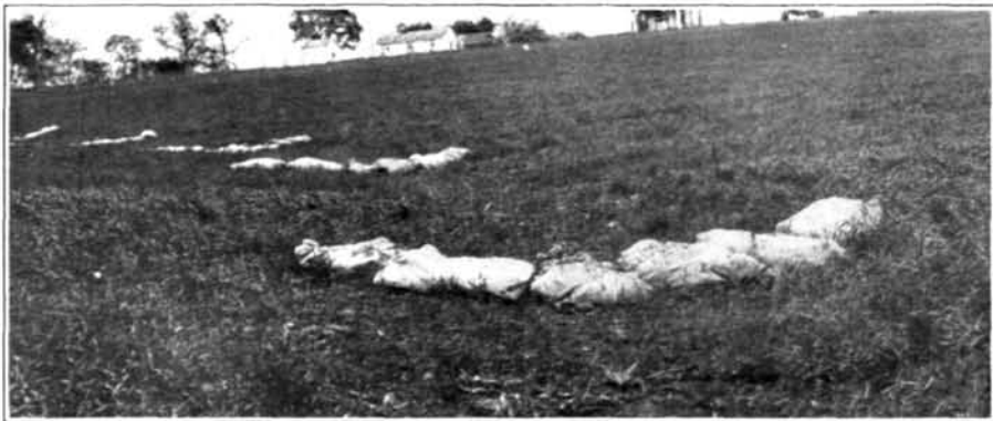
The formation of gullies can be checked by sodded dams constructed by placing burlap bags filled with sod in any depression which serves as a channel for conveying the runoff from a field terrace on a higher slope. This is a wide depression and thus required a great number of bags
