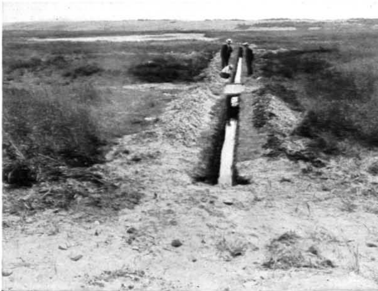
Swampy areas too extensive to permit filling in may be effectively rid of mosquitoes by means of properly constructed ditches. The main ditch for the area here shown is two miles long, draining at each end into a rocky beach.
