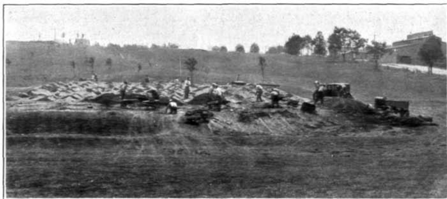
Rebuilding No. 1 putting green at the Audubon Country Club. On the second day of the work, after the old sod had been removed and proper tile drainage installed, a new 8-inch top soil is being prepared.
