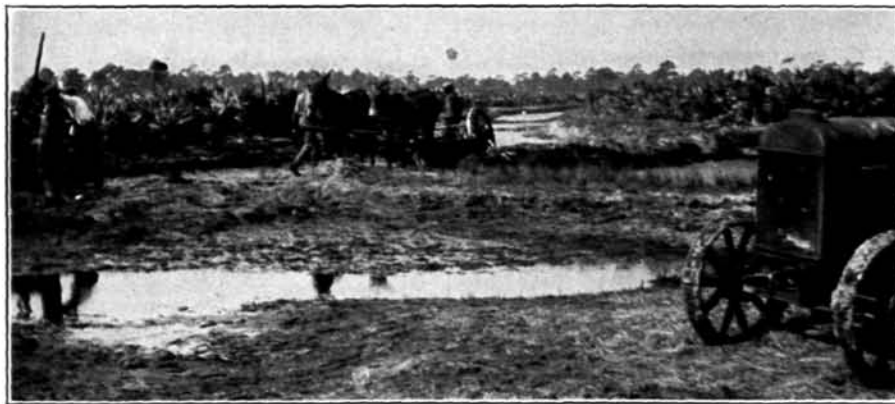
Digging a wide, open ditch with a wheel scraper on the side of a low fairway in Florida. The fill is being used to raise the fairway and to build the green and tee.
