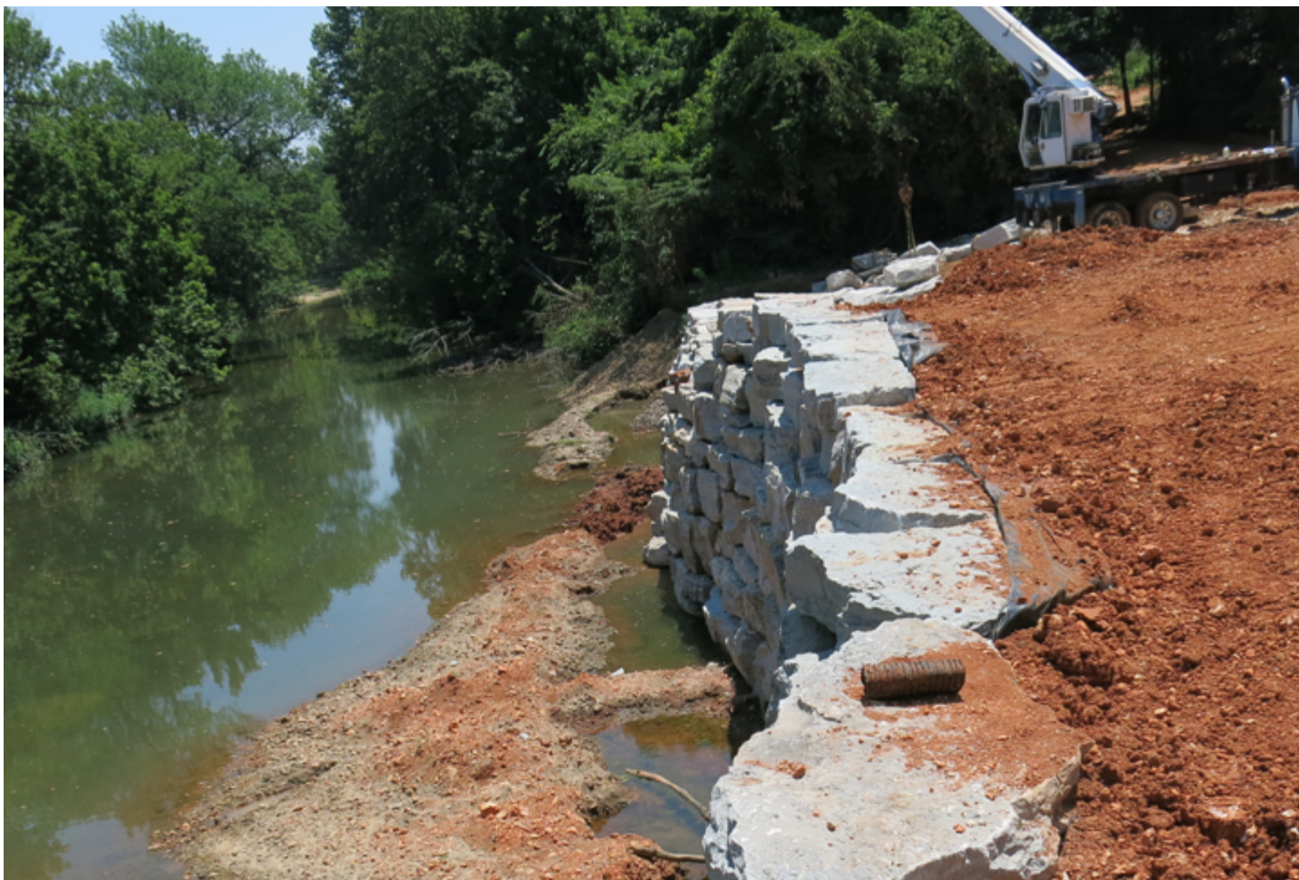
Areas adjacent to creeks and streams may need reinforcement to minimize the risk of future flood damage.
