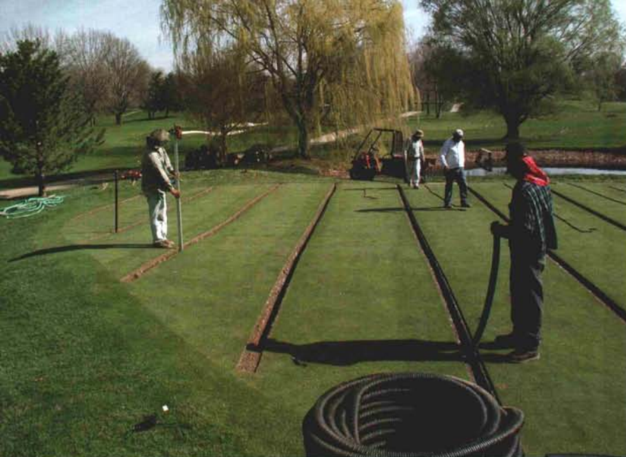
Subsurface drainage installation is tedious work that is often best left to the expertise of a drainage contractor.
