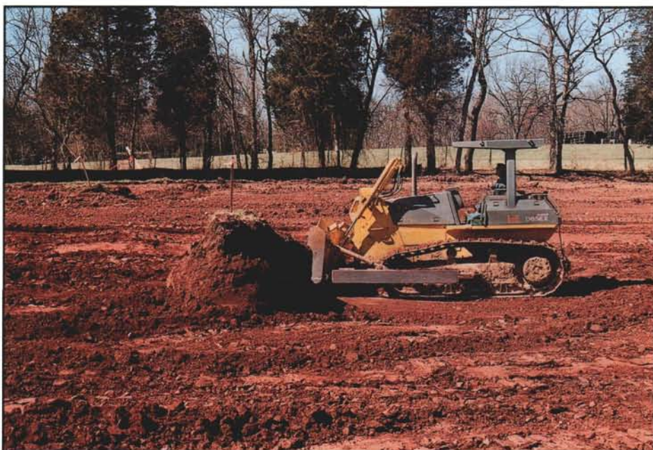
Heavy earth moving is expensive. This operator is making a cut of at least five feet.
