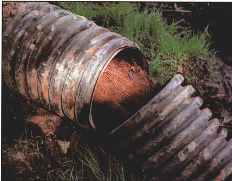
This 12-inch drainage pipe was filled with willow roots three months after installation.
