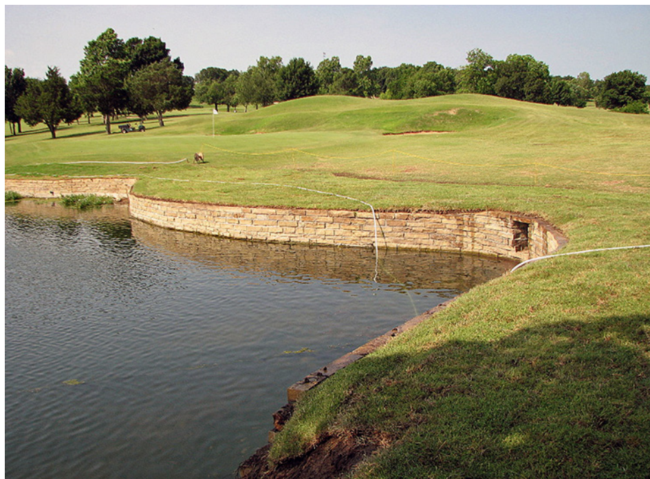
Retainer walls are projects often accomplished in-house, but the question should be asked, "Do they require engineering specifications to ensure adequate structural integrity?"
