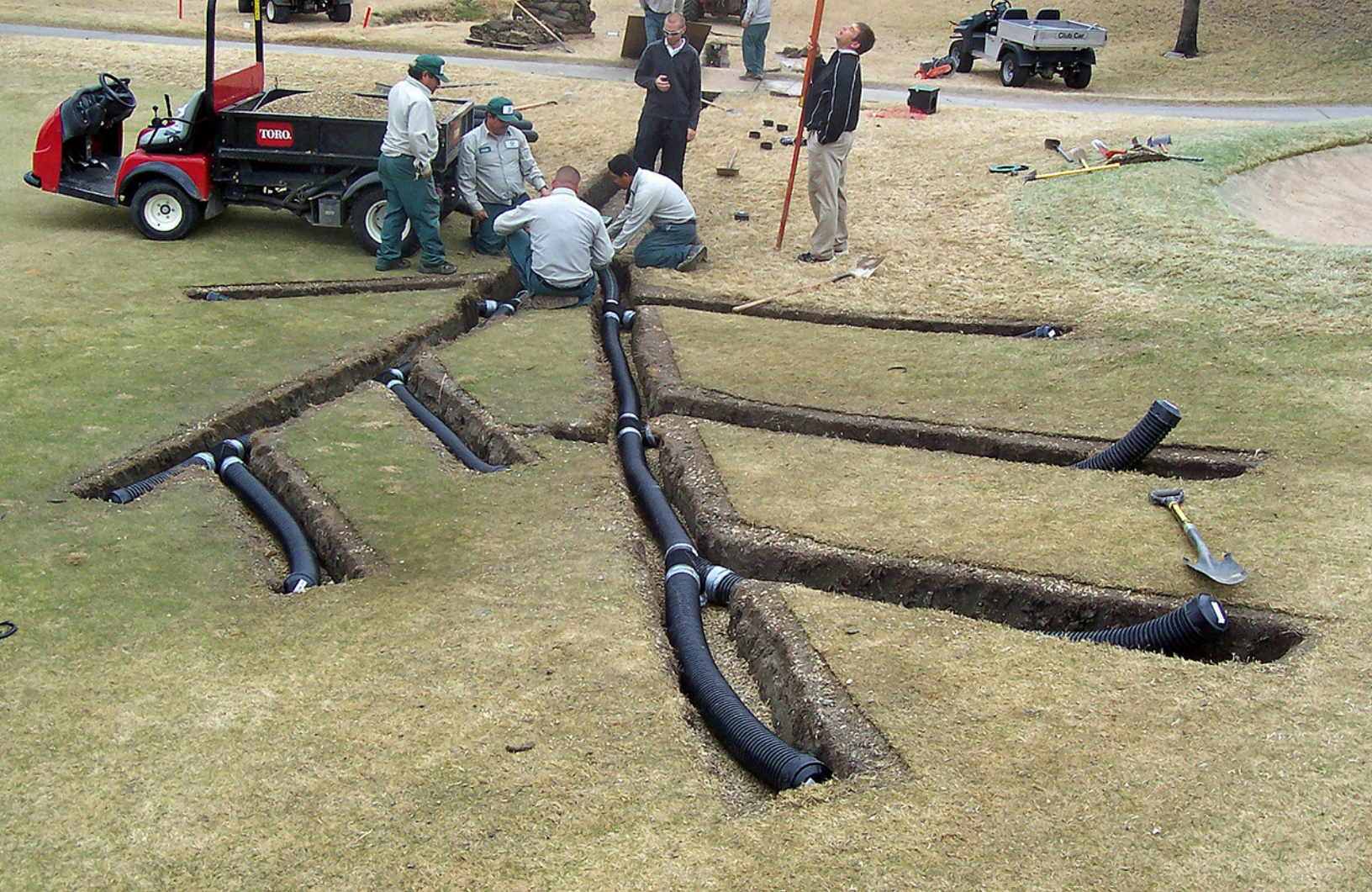
Winter drainage projects are one of the most common in-house projects completed by maintenance staff.
